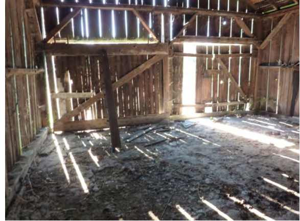
Image 139 - General deteriorated condition of slab and siding.
