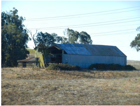
Image 57 – North side of Old Dairy Barn with collapsed section at east end
