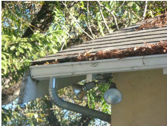
Image 34 - Debris filled gutter with new downspout
