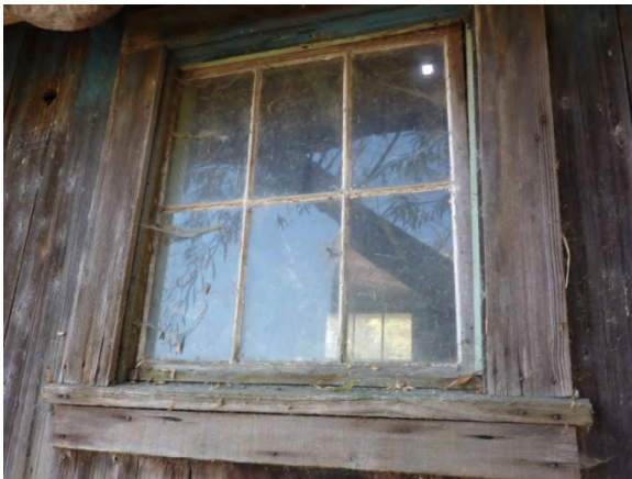
Image 100 - Deteriorated condition of window (typical)
