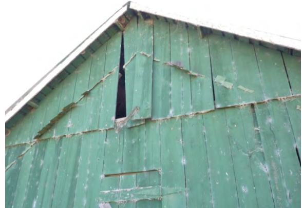
Image 137 - Typical condition of wood siding and vestiges of former addition east end.
