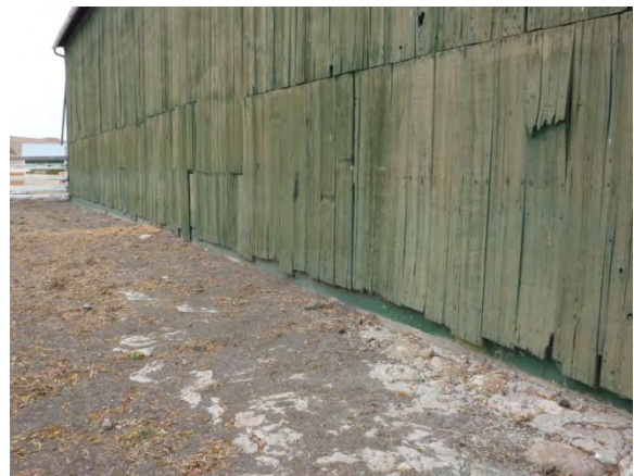
Image 51 - Typical repurposed and deteriorated siding
