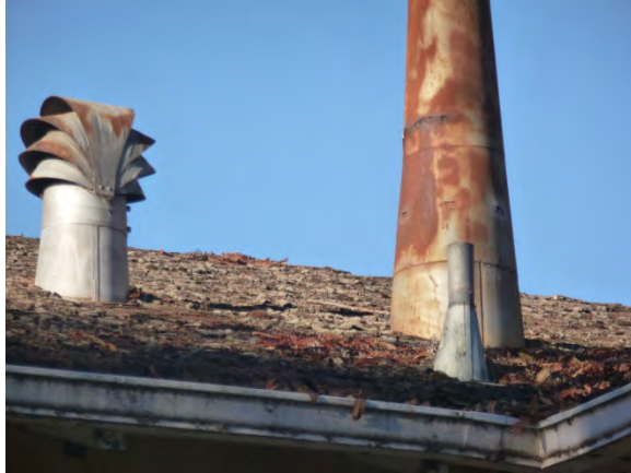
Image 33 - Deteriorated roofing and vents
