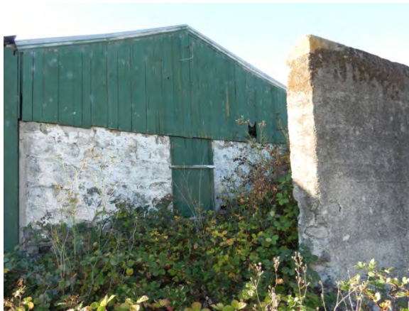
Image 73 - Overgrown vegetation on north side
