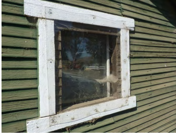
Image 111 - Poorly fit window with Plexiglas panel
