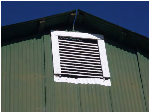
Image 53 – Gable vent with missing trim
