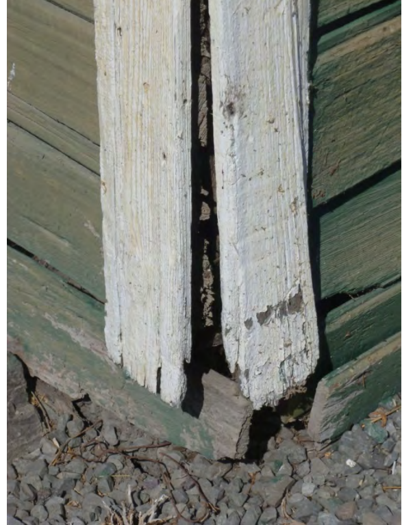
Image 110 - Deteriorated corner boards and earth to wood contact
