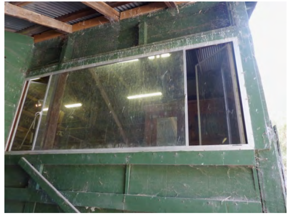
Image 91 - Poorly installed window adjacent to entrance.
