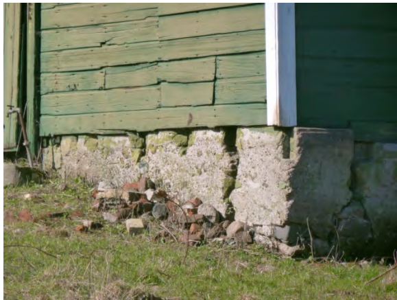
Image 70 - Failed wall at northeast corner
