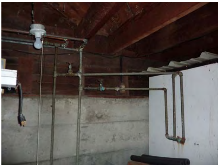
Image 44 - Deteriorated piping in basement
