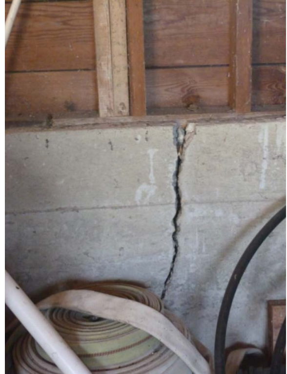
Image 26 - Structural crack in north wall
