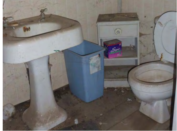
Image 95 - Deteriorated plumbing fixtures.
