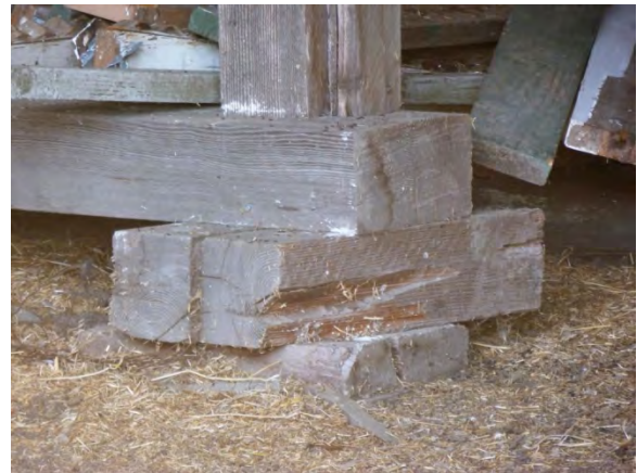
Image 60 - Wood framing resting directly on grade
