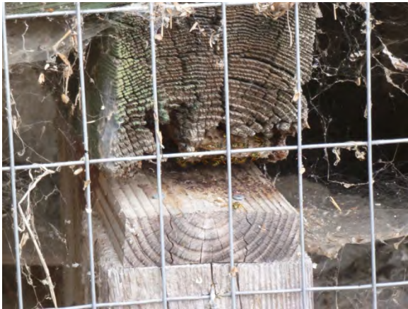
Image 84 - Deteriorated structure below building
