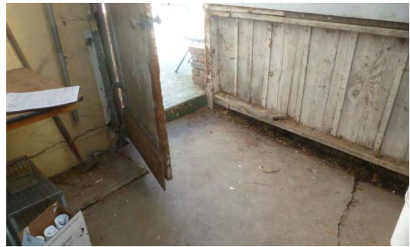
Image 39 - Deterioration in outdoor storage shed
