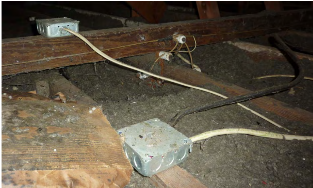
Image 24 – Mix of knob and tube and newer wiring in attic
