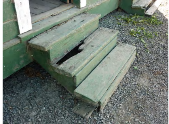
Image 112 - Deteriorated wood stairs directly on ground
