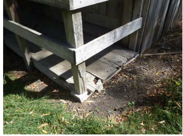
Image 101 - Deterioration at west end of porch
