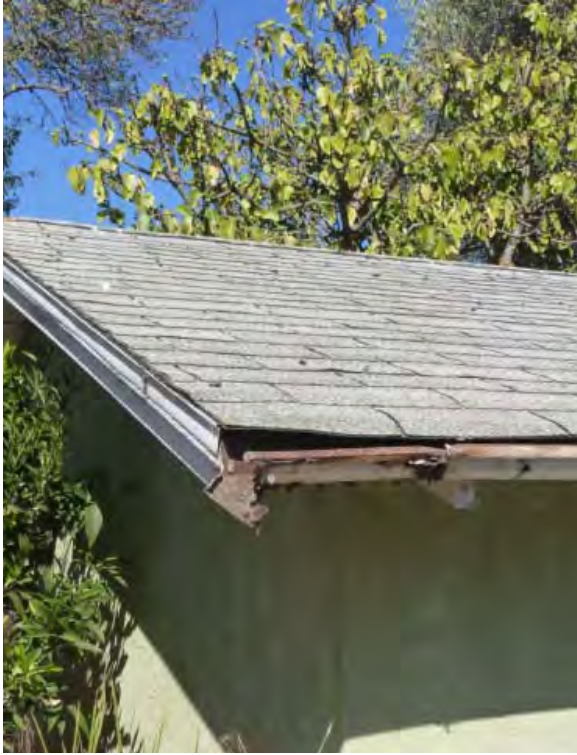
Image 25 - Garage roof and corroded gutter
