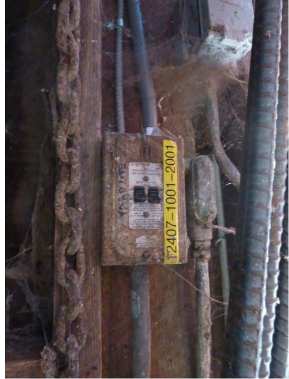
Image 121 - Corroded electrical components
