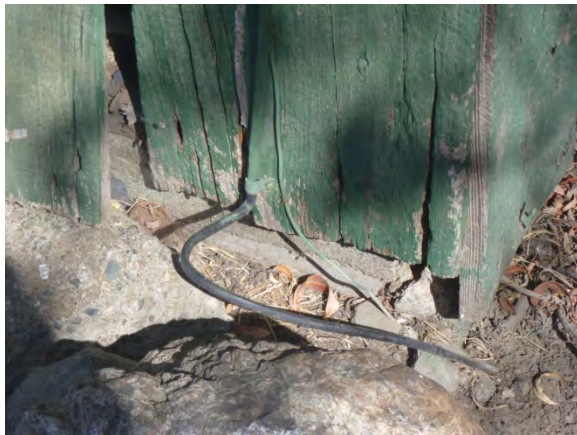
Image 127 - Deteriorated siding with wood to earth contact.
