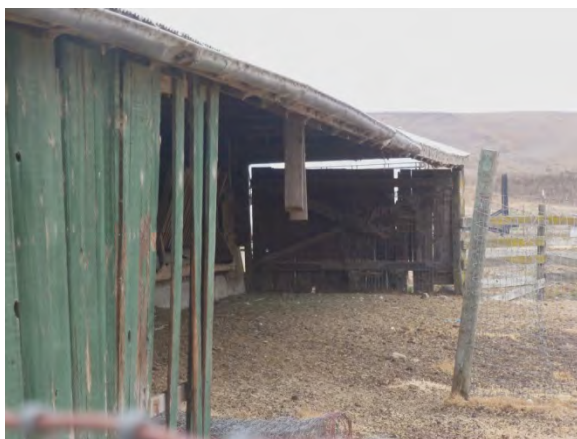
Image 50 - Failing roof at shed
