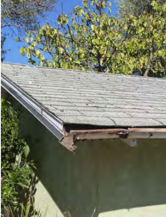
Image 25 - Garage roof and corroded gutter
