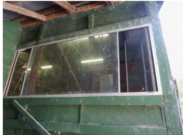
Image 91 - Poorly installed window adjacent to entrance.
