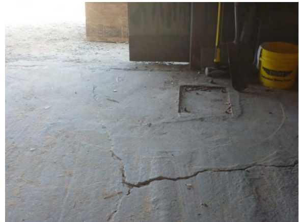
Image 130 - Cracked concrete slab
