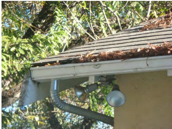
Image 34 - Debris filled gutter with new downspout
