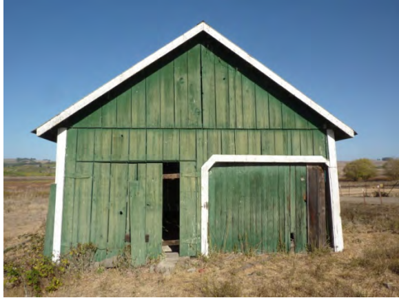
Image 138 - Non-functional doors at west wall.
