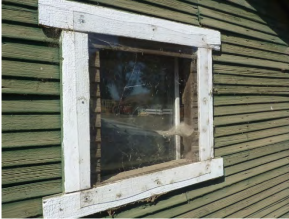
Image 111 - Poorly fit window with Plexiglas panel
