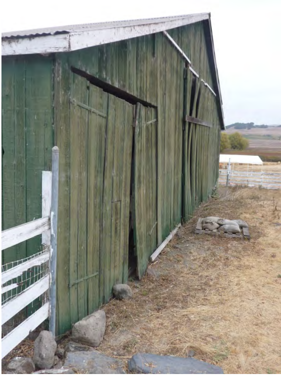
Image 118 - Deteriorated doors at south end of building
