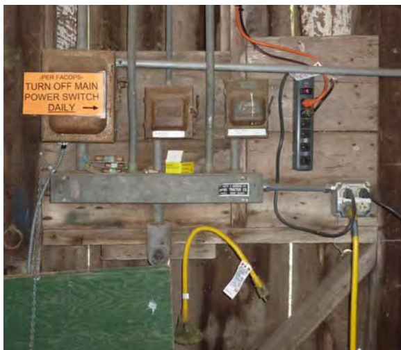
Image 131 - Miscellaneous non-compliant electrical modifications
