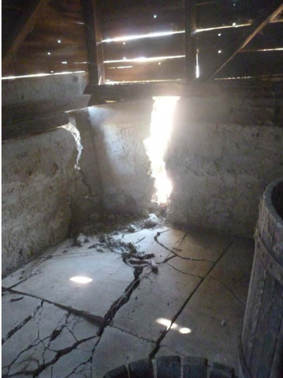
Image 77 - Condition at northeast corner.
