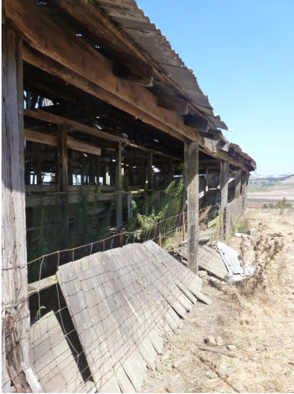
Image 61 - Failed wall at south side
