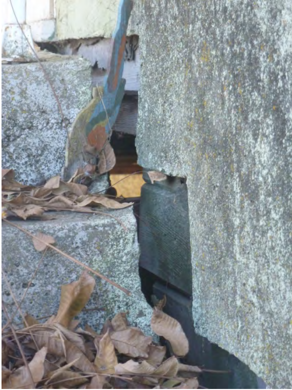
Image 19 - Front porch separated from wall of house
