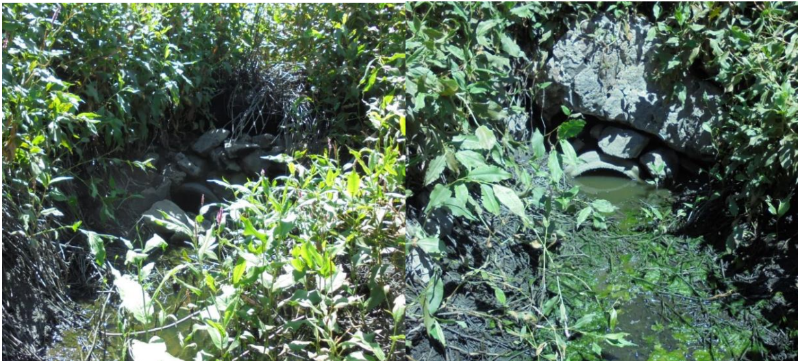
Figure 3. Largely blocked culvert in Causeway, inlet shown on left, outlet shown on right.
