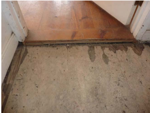
Image 40 - Flooring deterioration and change of level
