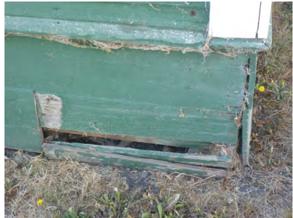
Image 6 - Typical wood to earth contact
