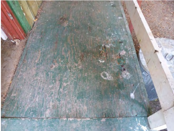
Image 92 - Deteriorated plywood at ramp to west entrance.
