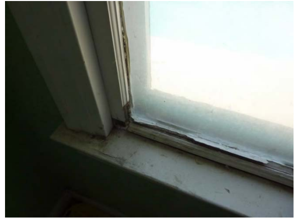
Image 42 - Deteriorated window at west wall
