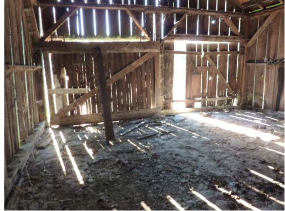
Image 139 - General deteriorated condition of slab and siding.
