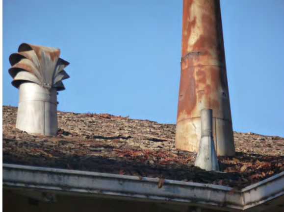
Image 33 - Deteriorated roofing and vents
