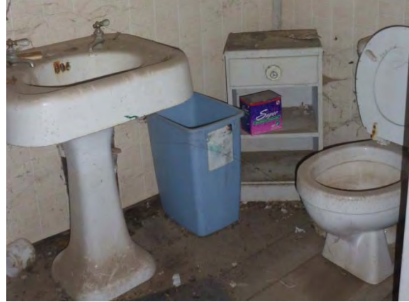
Image 95 - Deteriorated plumbing fixtures.
