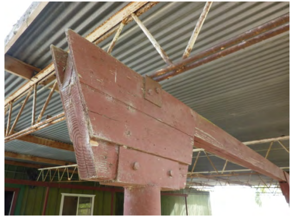
Image 85 - Deteriorated roof structure over picnic area
