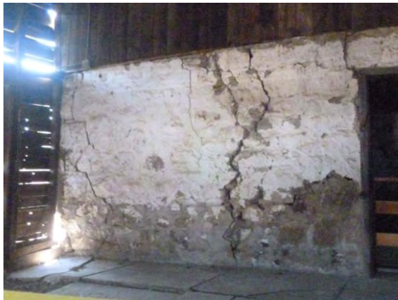
Image 69 - Severe cracking of masonry wall
