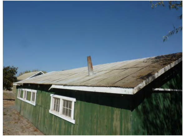
Image 123 – West wall and rusted roof of Storage Shed
