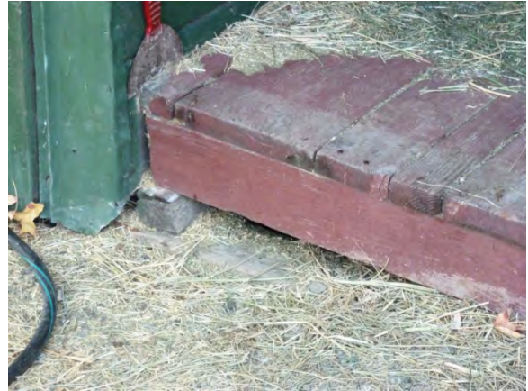
Image 93 - Wood to earth contact at stairs to north entrance.
