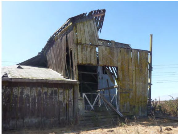
Image 59 - Collapsed east end of barn
