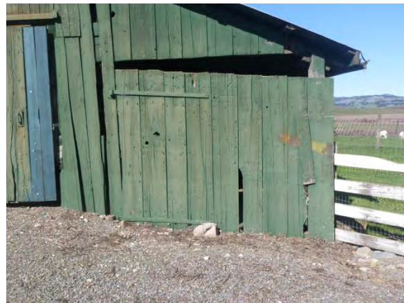
Image 52 - Shed siding with wood to earth contact
