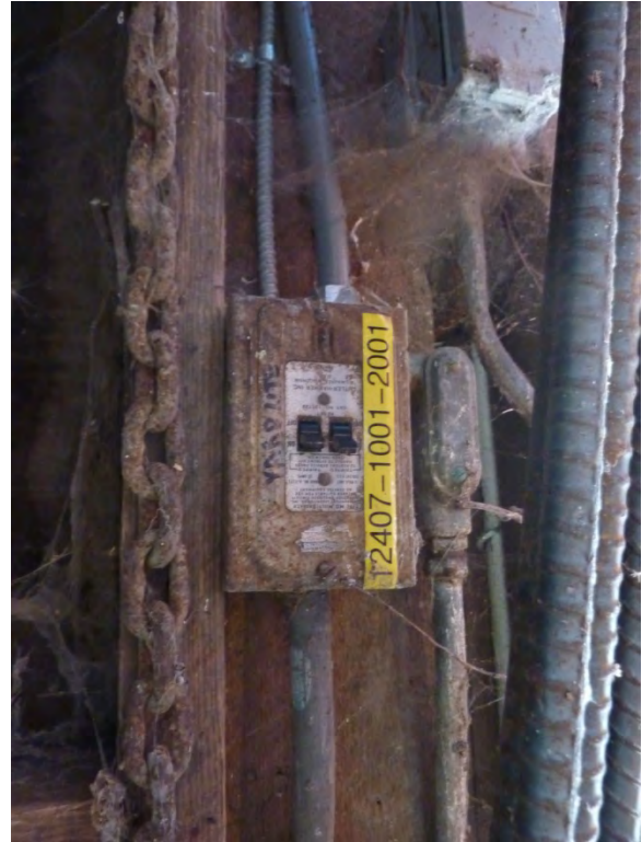
Image 121 - Corroded electrical components
