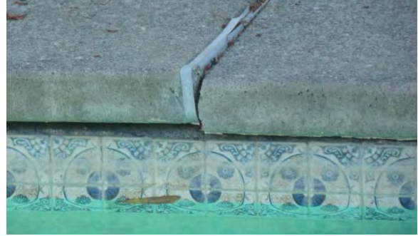
Image 38 - Misaligned paving at pool
