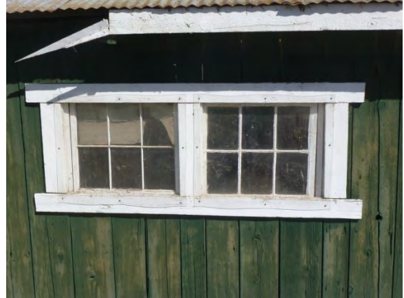
Image 128 - Typical window with Plexiglas covering; damaged trim
