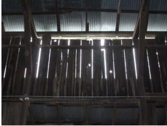
Image 55 - Interior view showing condition of siding
