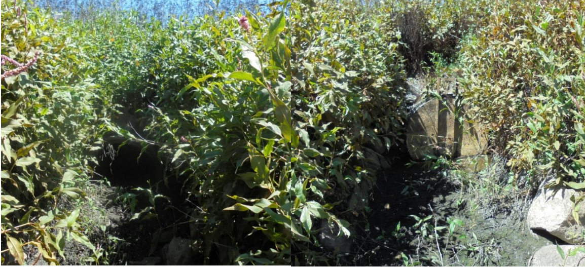
Figure 4. Closed gated culvert in horseshoe berm, inlet shown on left, outlet shown on right.
