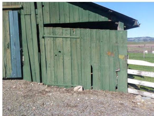
Image 52 - Shed siding with wood to earth contact
