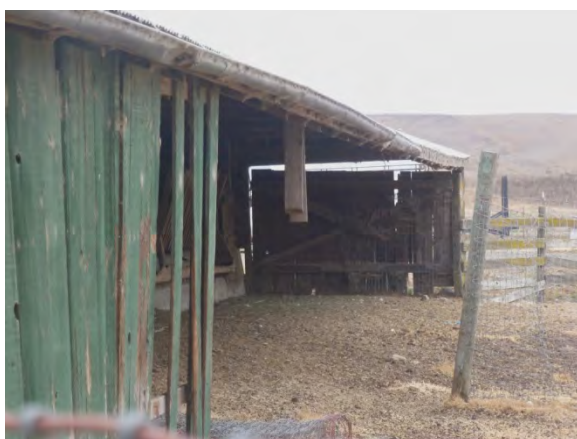
Image 50 - Failing roof at shed
