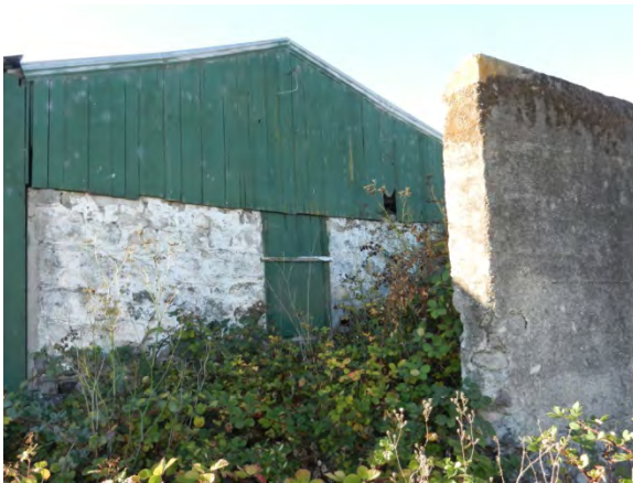
Image 73 - Overgrown vegetation on north side
