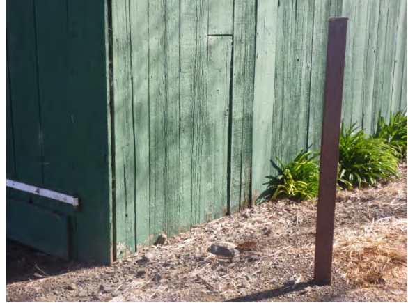
Image 117 - Wood to earth contact of siding
