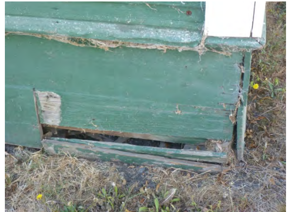
Image 6 - Typical wood to earth contact
