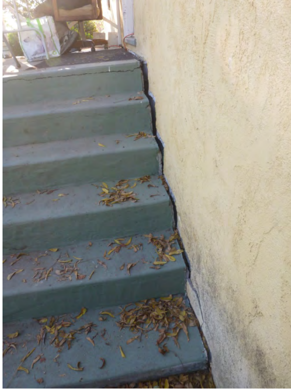
Image 37 - Front porch stair separated from house wall
