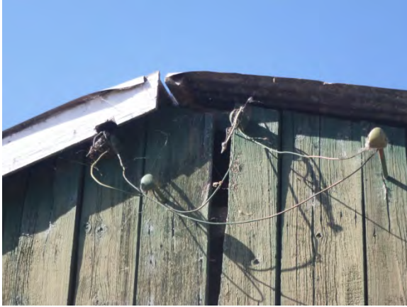
Image 72 - Condition at ridge
