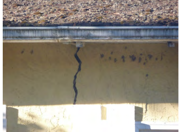
Image 35 - Crack in east wall at addition
