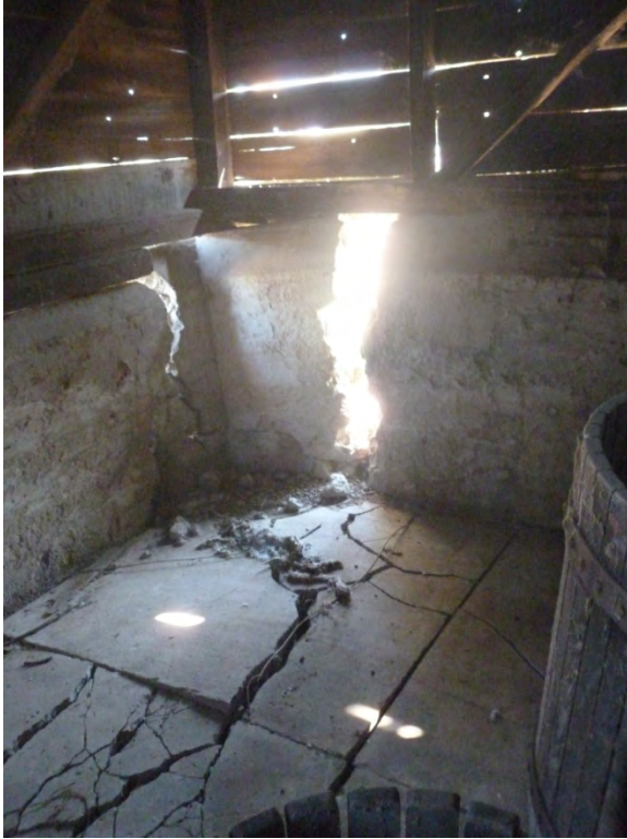
Image 77 - Condition at northeast corner.
