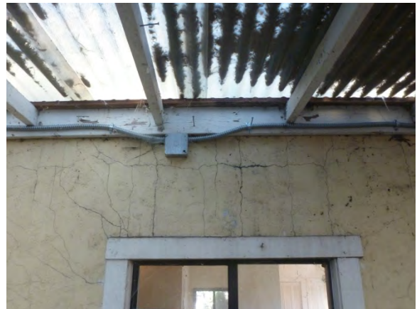
Image 36 - Extensive cracking at south wall
