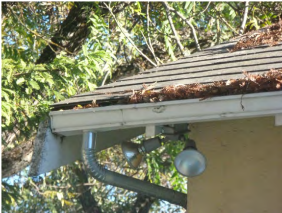
Image 34 - Debris filled gutter with new downspout
