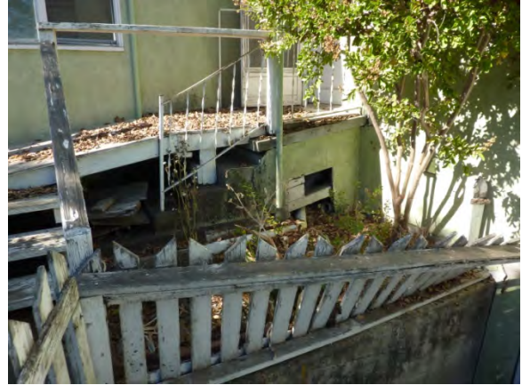
Image 20 - Poorly constructed ramp and stairs at south entrance
