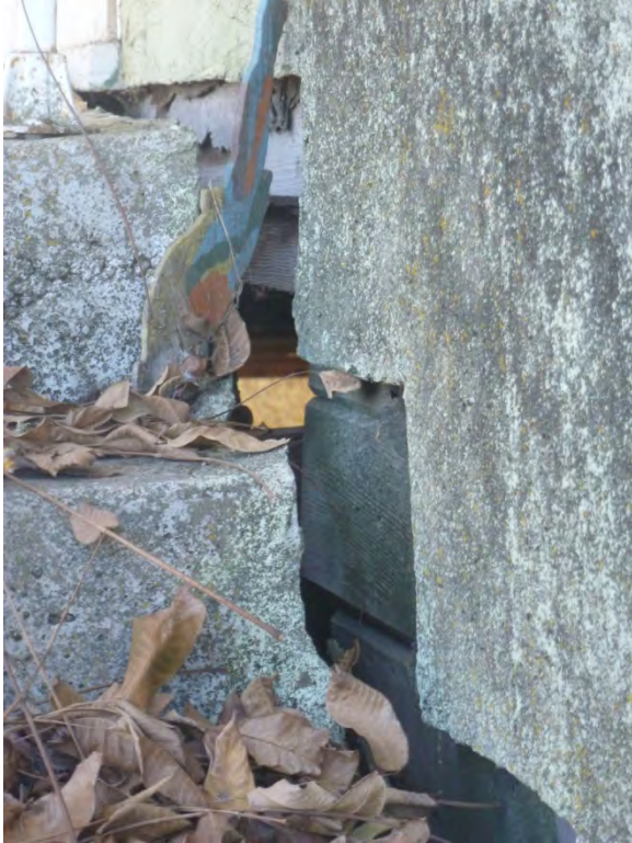
Image 19 - Front porch separated from wall of house
