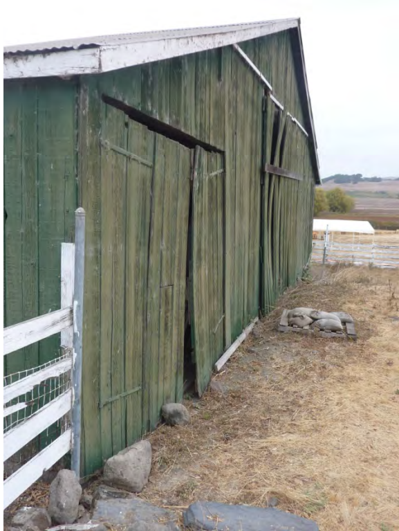
Image 118 - Deteriorated doors at south end of building
