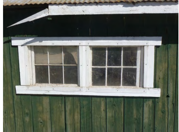
Image 128 - Typical window with Plexiglas covering; damaged trim
