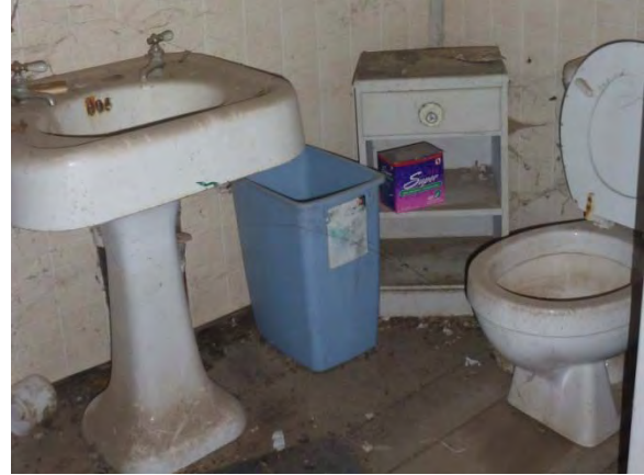
Image 95 - Deteriorated plumbing fixtures.
