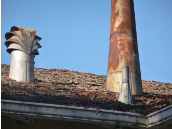
Image 33 - Deteriorated roofing and vents
