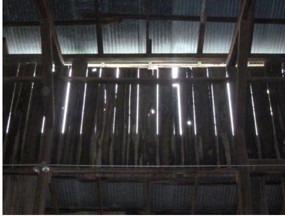
Image 55 - Interior view showing condition of siding
