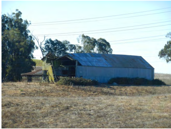
Image 57 – North side of Old Dairy Barn with collapsed section at east end
