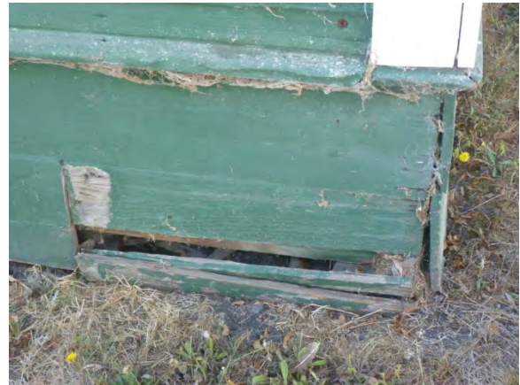
Image 6 - Typical wood to earth contact
