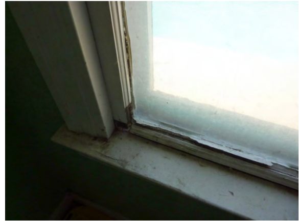
Image 42 - Deteriorated window at west wall
