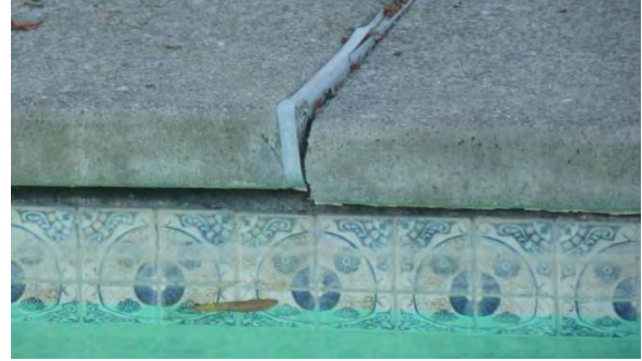
Image 38 - Misaligned paving at pool
