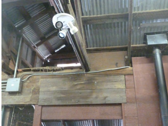
Image 94 - Typical electrical installation.
