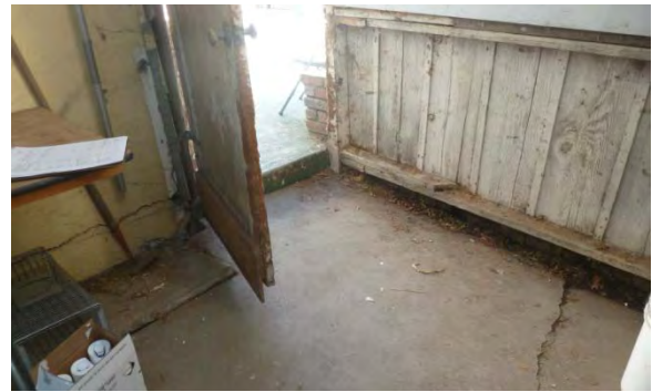
Image 39 - Deterioration in outdoor storage shed
