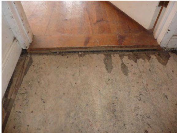
Image 40 - Flooring deterioration and change of level
