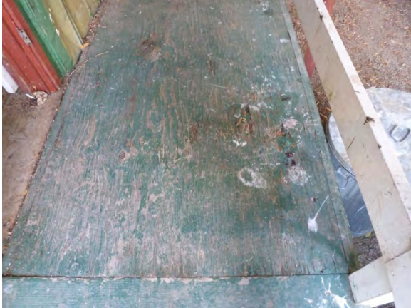
Image 92 - Deteriorated plywood at ramp to west entrance.
