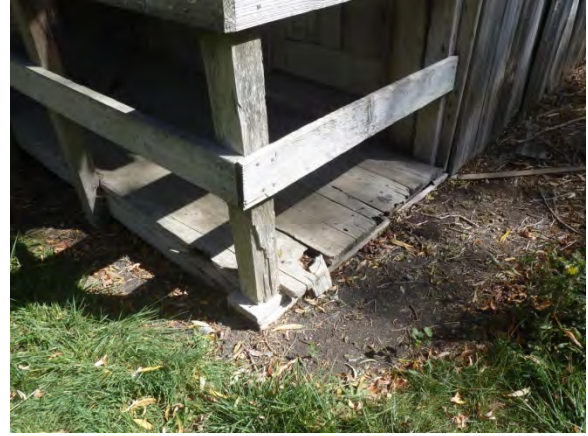
Image 101 - Deterioration at west end of porch
