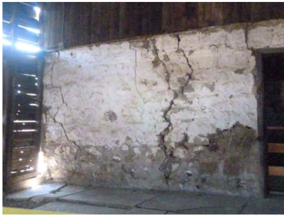
Image 69 - Severe cracking of masonry wall
