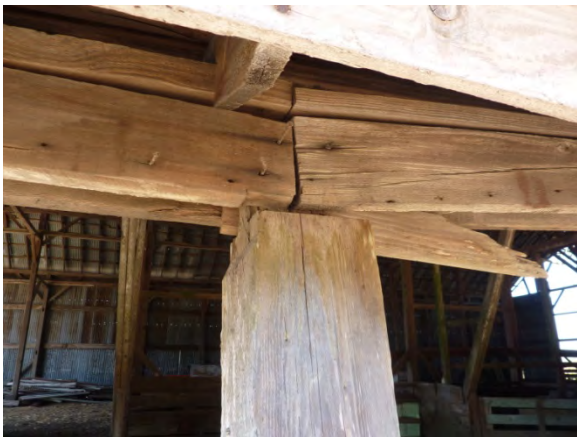
Image 62 - Structural Damaged at south wall
