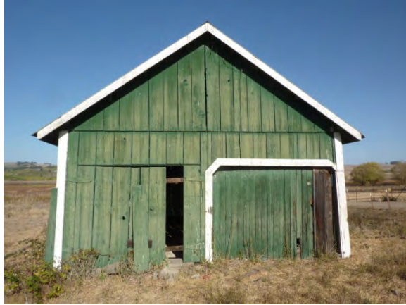
Image 138 - Non-functional doors at west wall.
