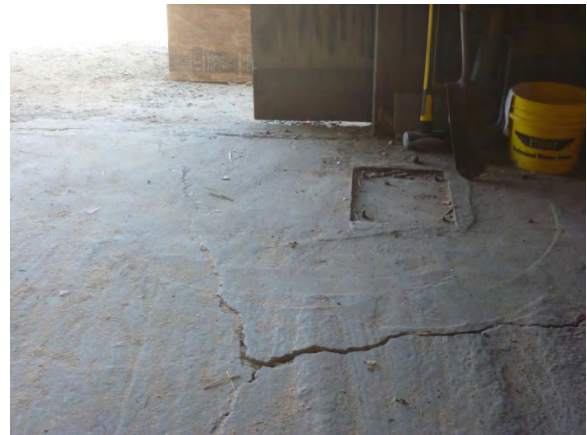
Image 130 - Cracked concrete slab
