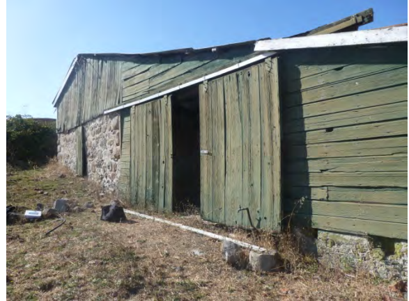
Image 74 - South wall showing poor overall condition of siding and doors
