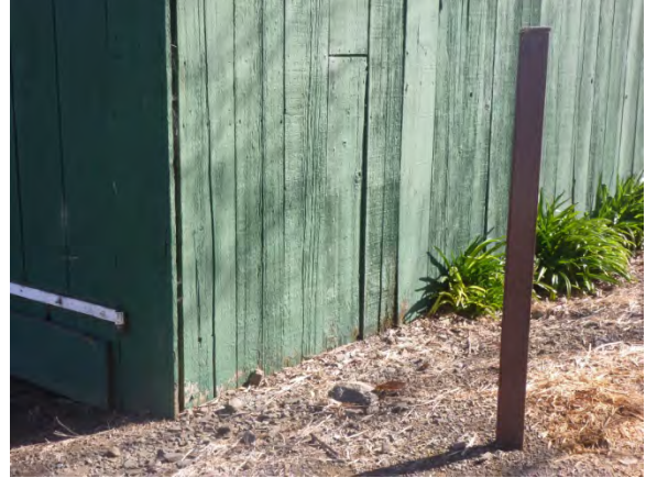
Image 117 - Wood to earth contact of siding
