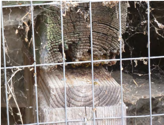
Image 84 - Deteriorated structure below building
