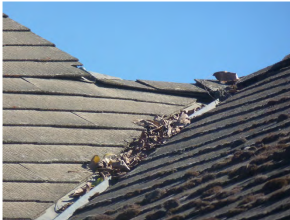
Image 17 - Deteriorated shingles and debris
