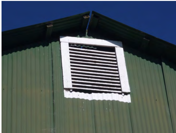
Image 53 – Gable vent with missing trim
