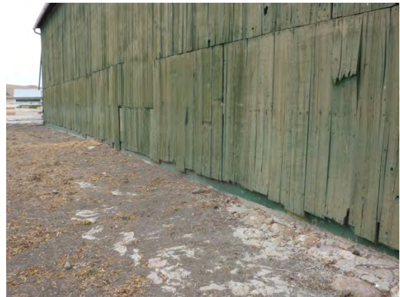
Image 51 - Typical repurposed and deteriorated siding
