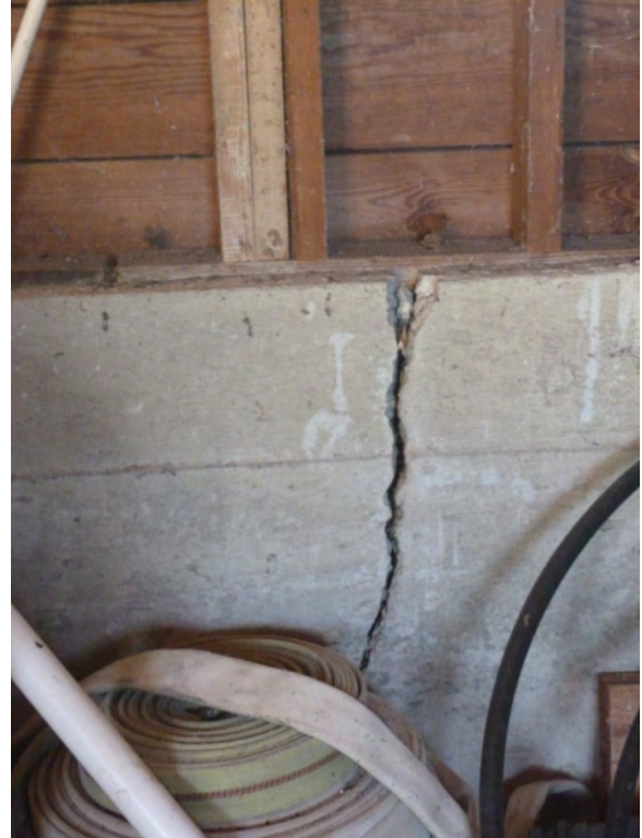
Image 26 - Structural crack in north wall
