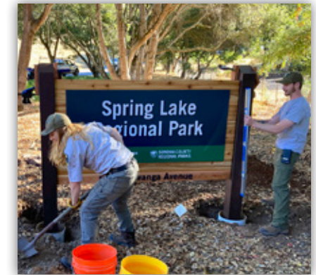
A Regional Parks crew installs a new sign at Spring Lake Regional Park.
